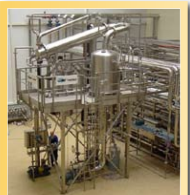
Deaerator and Deoiler
