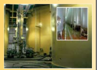
Aseptic Tanks Farm NFC capabilities
